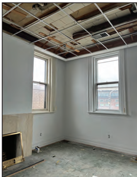
Renovations are underway to the Cathedral Convent building in Scranton, which will soon be the Saint Pius X Seminary. The updates include new carpet, light fixtures and paint.
