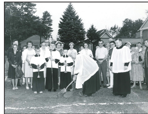
Rev. Thomas P. Monahan breaks ground for a convent on Saint Aloysius Church property on August 23, 1962. The convent was built to care for the Sisters of Mercy stationed at Saint Aloysius.
