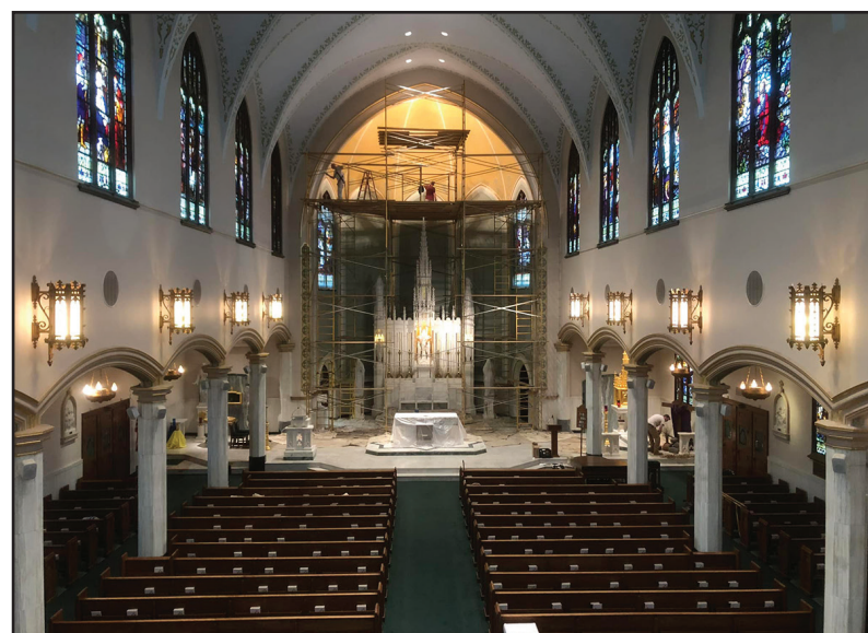
In advance of its 125th anniversary Mass, 42-foot-tall scaffolding has been temporarily put up inside Saint Aloysius Church so that the sanctuary area of the church can be painted by Robert A. Ritterbeck Painting, Inc.
